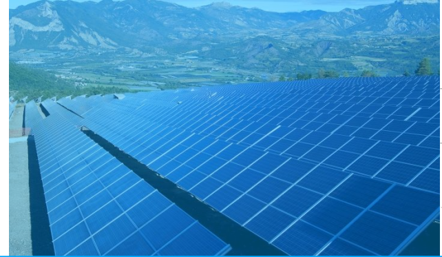
Centrale photovoltaïque - Ourbans, France
